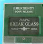
Emergency Break Glass
